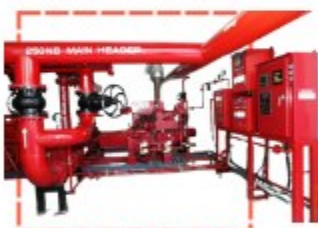
Hydrant Center Pump
