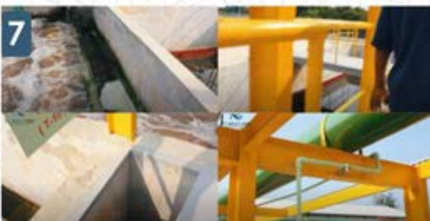
7 Gutter, Septic Tank, Effluent Tank, Inject Chlorine
