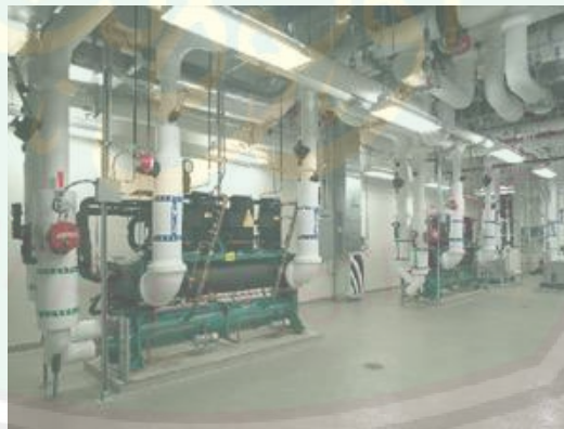
Gambar 2. 26 Ruang Chiller (Sumber: http://www.acrokool.com.au/acro2015/images/chillers-room-service-product-4.jpg )
