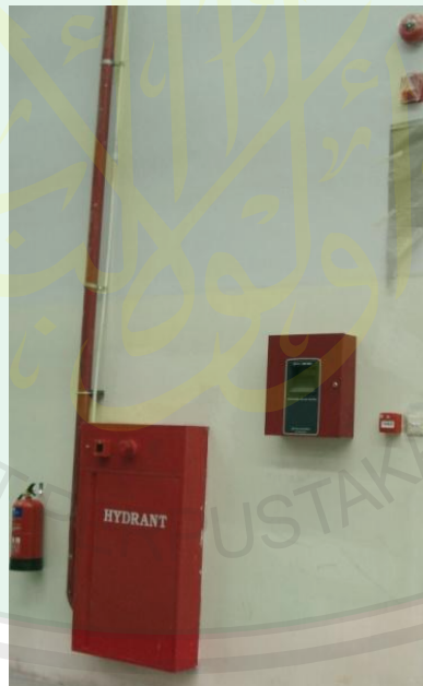
Gambar 4.86 indoor hydrant box (Sumber: Hasil Analisis. 2010)
