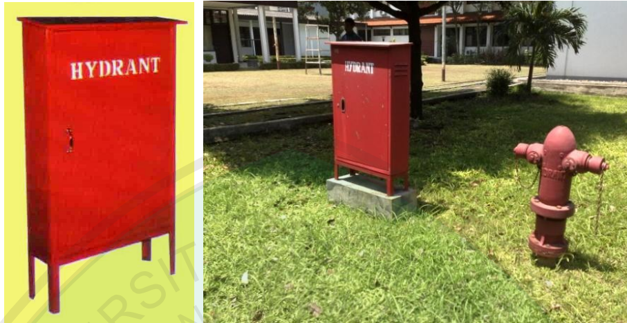
Gambar 4.87 outdoor hydrant box (Sumber: Hasil Analisis. 2010)
