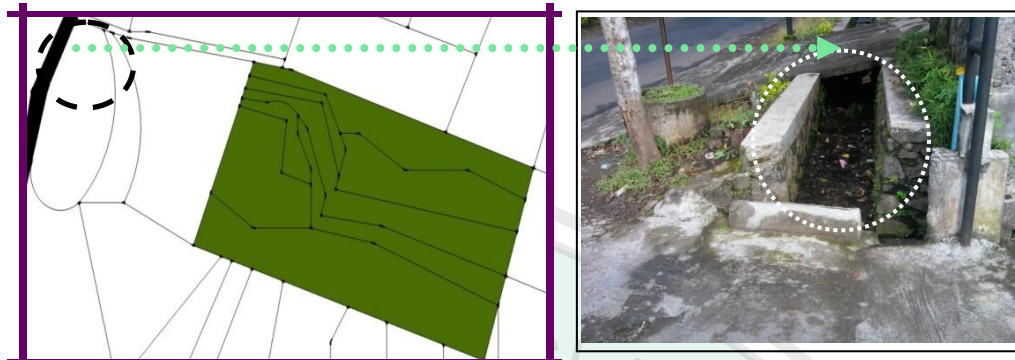
Gambar 4.11 Drainase Sumber : Hasil survey (2012)
