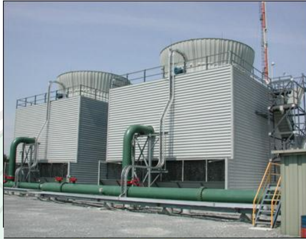
Gambar 4.98 cooling tower Sumber : www. google.co.id (2013)
